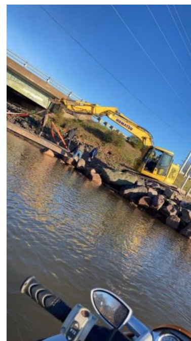
The excavator on the slipway lifting the docks back (this photo shows the height of the water at normal high tide)
